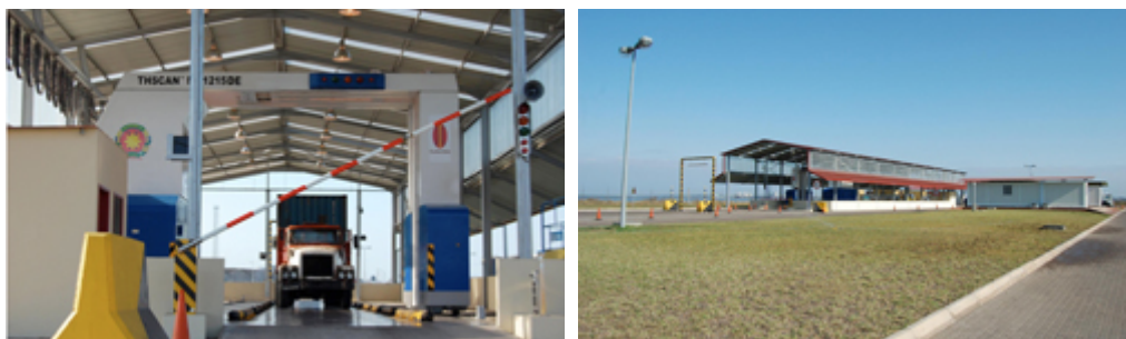
Radiation Monitor (RM2000), X-Ray Scanner, MB1215DE, 6 MeV, Dual Power System, installed at the Port of Maputo (since July 2009)
