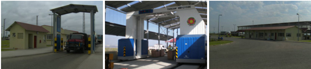
Radiation Monitor (RM3000), X-Ray Scanner, MB1215DE, 6 MeV, Power System and INI facilities at the Port of Beira
